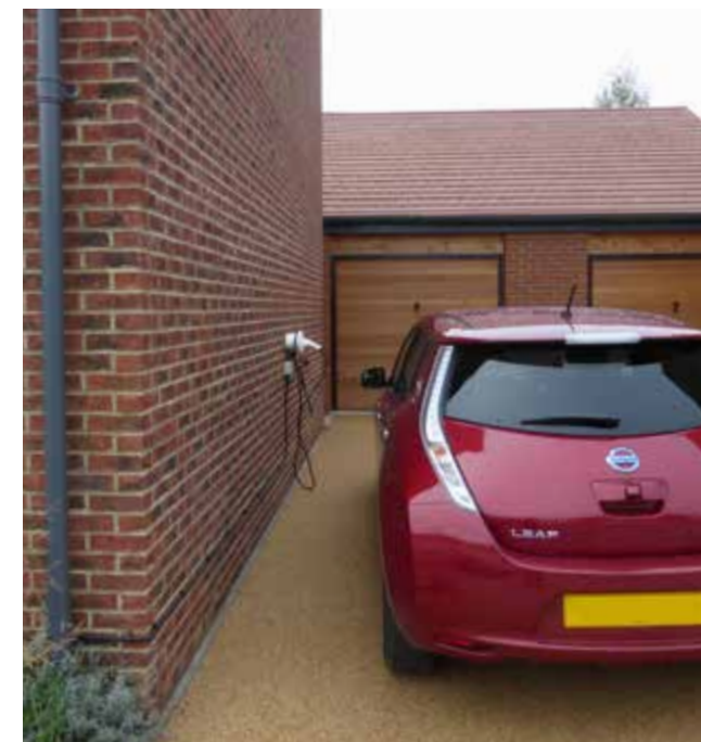
Home electric vehicle charging
